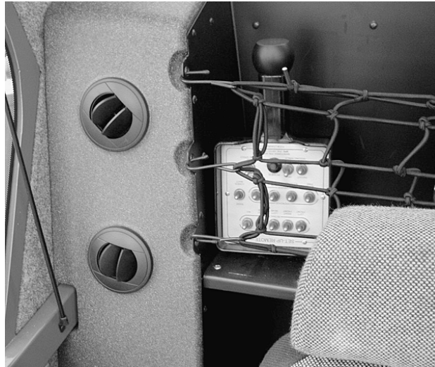
Remote Control Stored on Shelf Behind Seat in Cab
