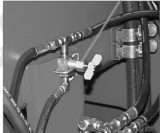
View Between Rear Drum and Hydraulic Tank
