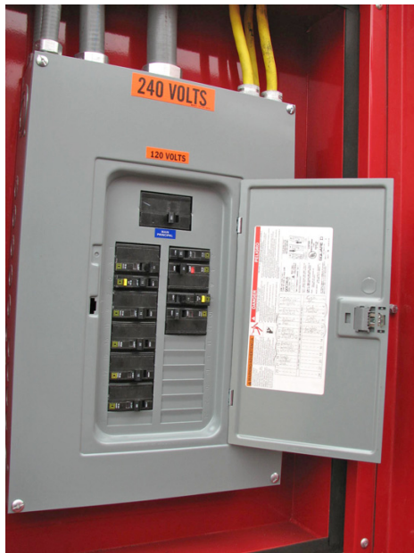
Main Load Center Circuit Breakers
