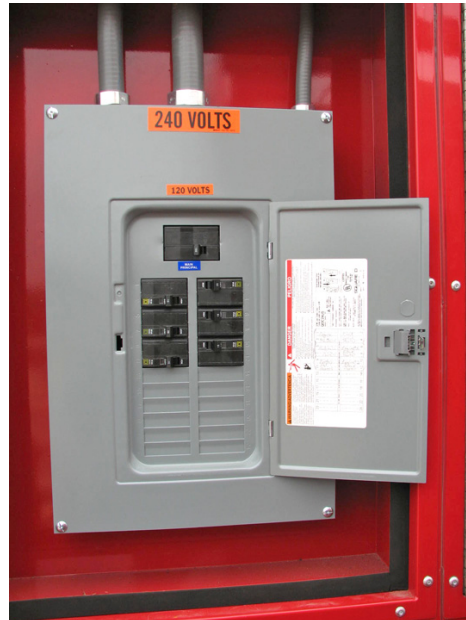
Cold Weather Load Center Circuit Breakers
